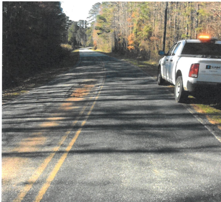
Alligator Cracking (Patch and Overlay)
